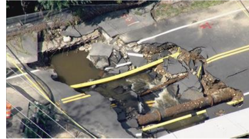
Washed out road in Leominster, CBS Boston September 2023
