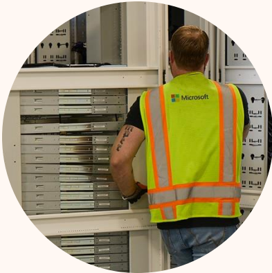
Datacenter efficiencies & innovation
